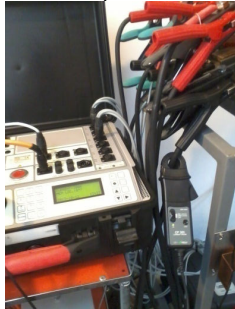
Figure 2.1 Measurement of the circuit breaker resistance with BSG using test device with the external current clamps
