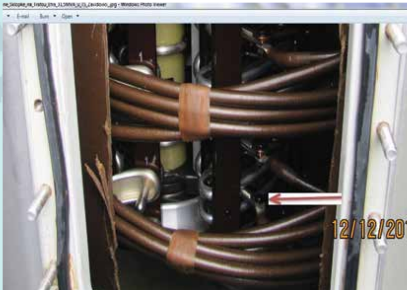
Figure 7: Exact Position of the Loose Bolt
